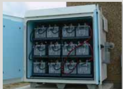
False River Regional Airport is the first airport in the U.S to have both taxiway and runway airfield lighting circuits on an APS system.
