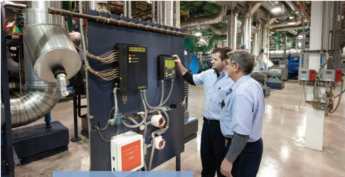
Operators reviewing refrigerant monitors.
