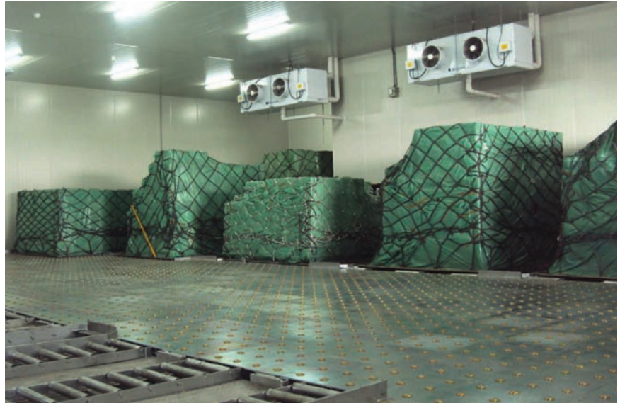
The Pharma Zone is a dedicated temperature-controlled handling facility for exporting pharmaceuticals. The facility features two cooling chambers with different temperatures – one for storing pharmaceuticals at a range of 15 degrees Celsius (59 degrees F) and 25 degrees Celsius (77 degrees F) and another for storing even more sensitive products at between 2 degrees Celsius (35 degrees F) and 8 degrees Celsius (46 degrees F). GMR Group
