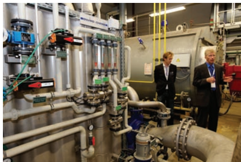
After the mechanical cleaning, the reclaimed deicing fluid is chemically cleaned with absorption and ion exchanger units.
