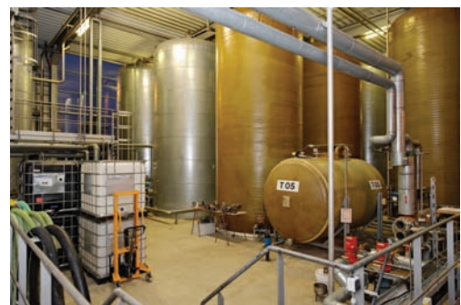
The reclaimed deicing fluid also goes through an evaporation unit to get rid of excess water and achieve the right concentration of glycol and, finally, an additive package is dosed into the fluid as its pumped into these batch tanks.
