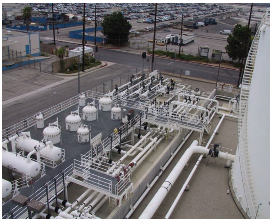
A series of pipelines receive fuel to the facility.
