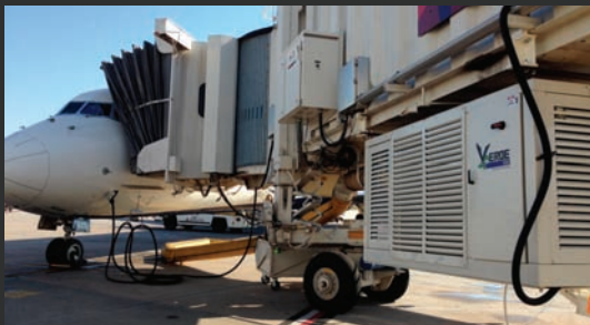
Verde 60 Ton bridge mount PCA system at Orlando International Airport
