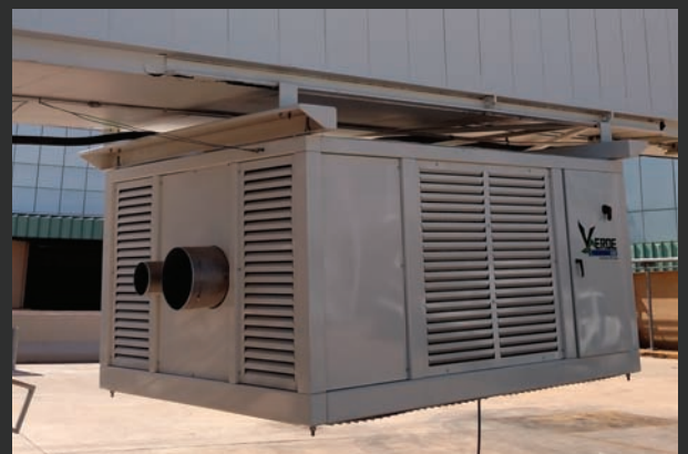
Verde 45 Ton Heat Pump PCA system at Louis Armstrong New Orleans International Airport
