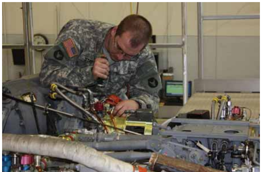
Technician Scott Staiert working on the upper-deck of a Black Hawk undergoing a Phase 2 inspection. Photo by Ronald Donner.
