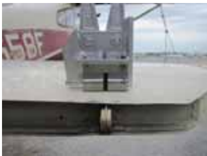
Thin skin damage on Cessna stabilizer straightened.
